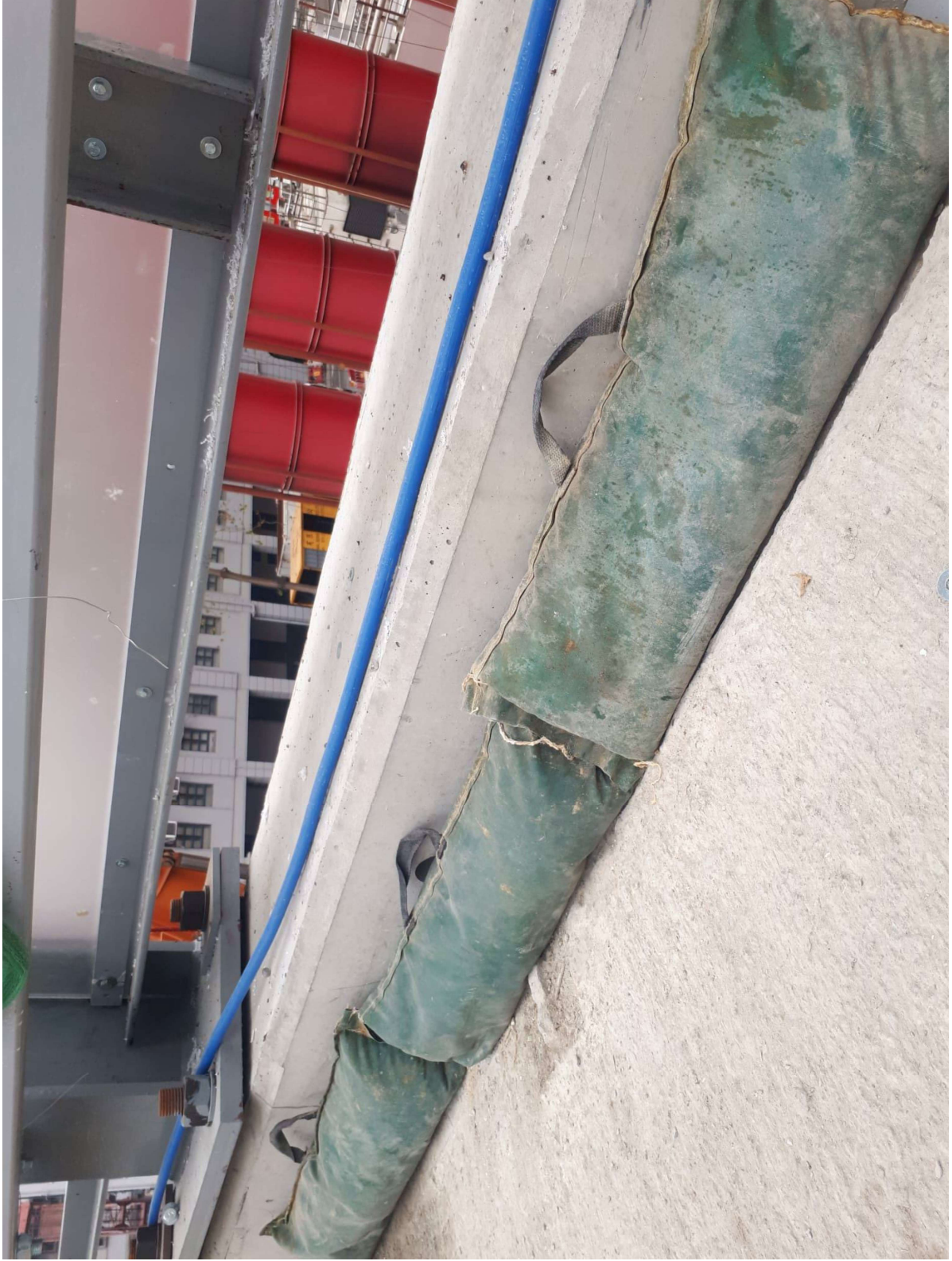
Remark 2: Bund along the bridge to prevent surface runoff outside the construction site
